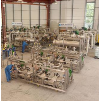
WFI & PW Distribution & POU
